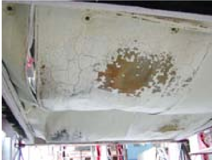
Figure 4.58: Suspended ceiling after test.
